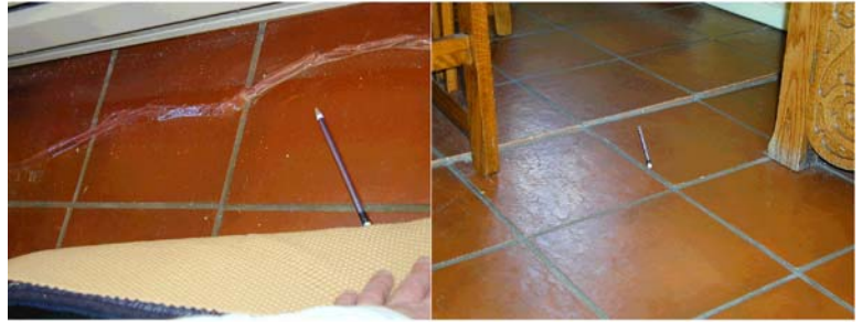
Crack and Raised Edge
