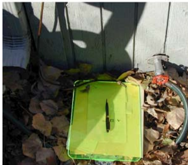
Missing drain line, unattached leg, Water
