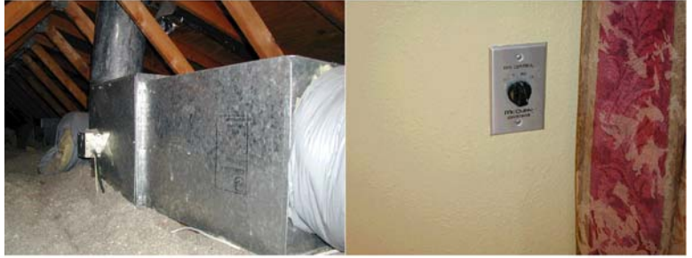
McQuay Air handler ????
