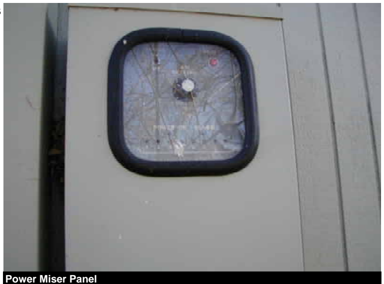
Power Miser Panel
