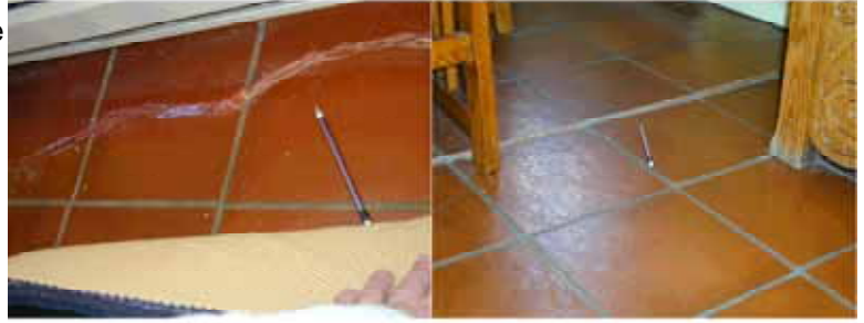
Crack and Raised Edge
