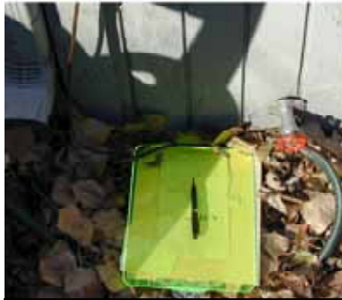
Missing drain line, unattached leg, Water
